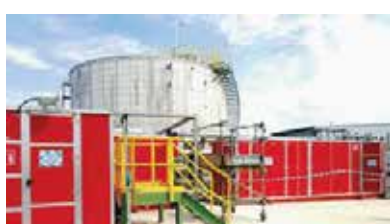
Fire Pumps for Refinery
